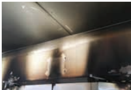
Photo 4: The HOT ROD Compressible Firestopping on the non-fire side. Although the double metal door failed and allowed fire and smoke to pass through the door, fire or smoke was unable to pass through the head-of-wall joint as indicated in the clean, off-white seal between the ceiling and the wall.
