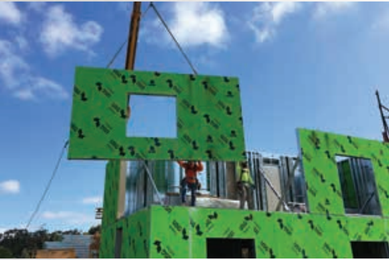
Photo 1: A six-story building was panelized and erected on a shake table at UCSD.
