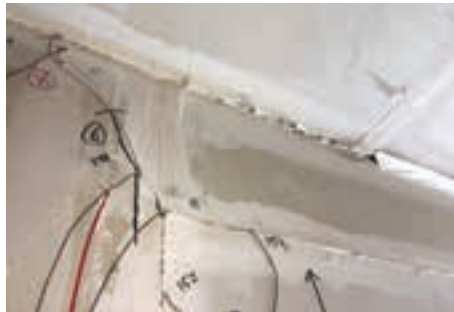
Photo 3: The results of the traditional method at the non-fire side where the paper tape cracks and pulls apart, which, in return, allows smoke to pass through the head-of-wall joint.
